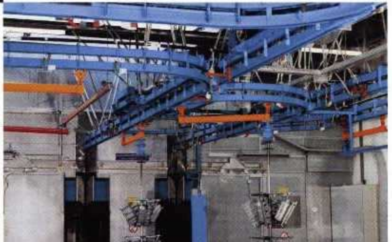
Blast cleaning of aluminium parts on a Power and Free system C10530
